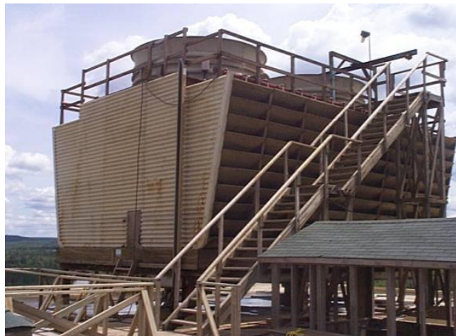
A cooling tower may be found on your school's roof or outside next to the HVAC room.
