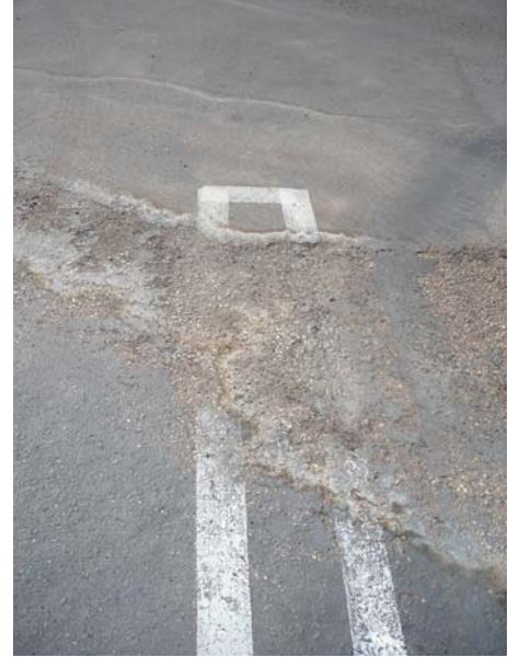
Paved areas such as parking lots and sidewalks can become damaged by runoff.
